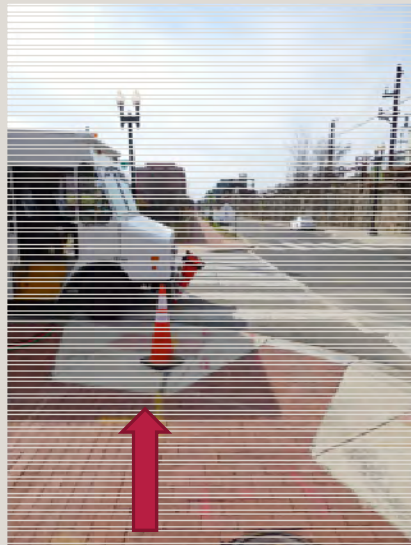
Maintaining ADA accessibility
