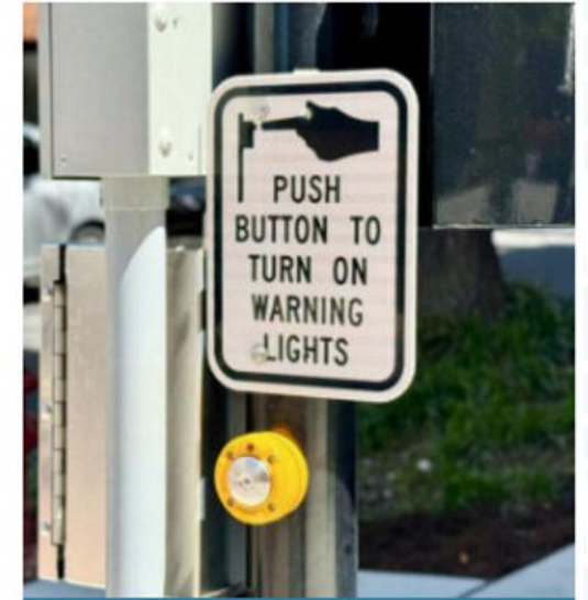
Rapid Flashing Beacons
