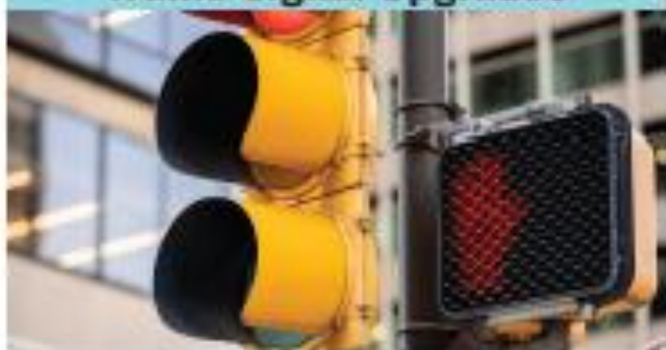
Traffic Signal Upgrades
